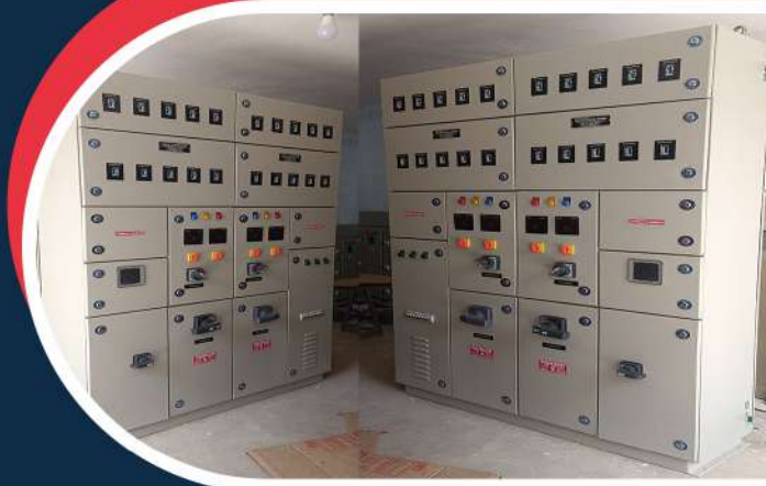
Function hall panel boards
