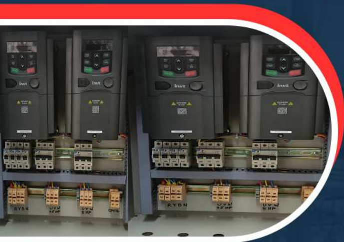
Drive panel boards
