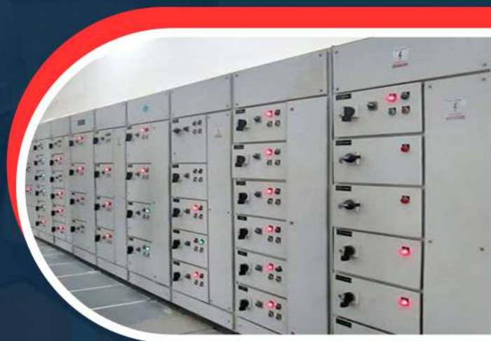
Mcc panel boards
