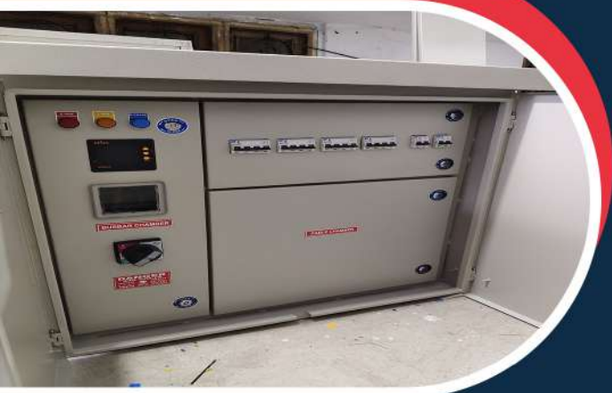
Out door panel boards
