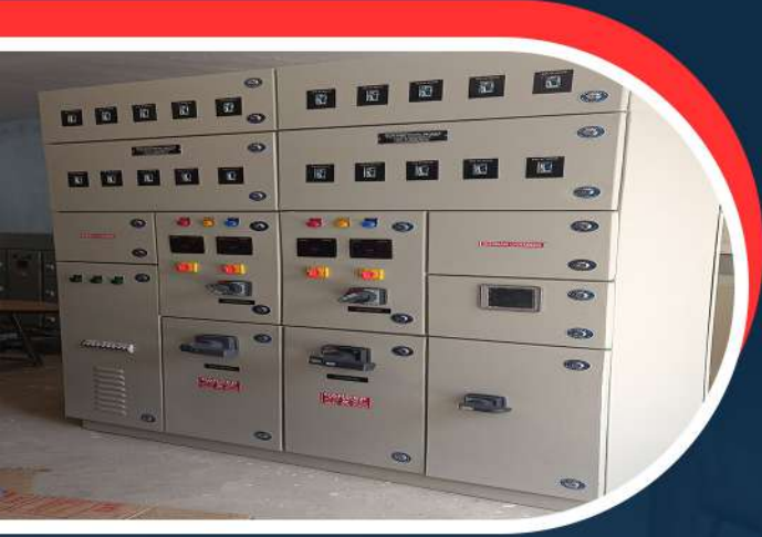
Function hall panel boards
