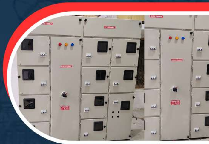
Meter panel boards
