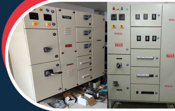
Pcc panel boards
